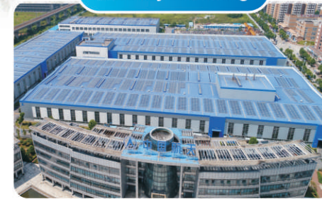
Aerospace Cable Photovoltaic Power Generation Project, Huangshi
